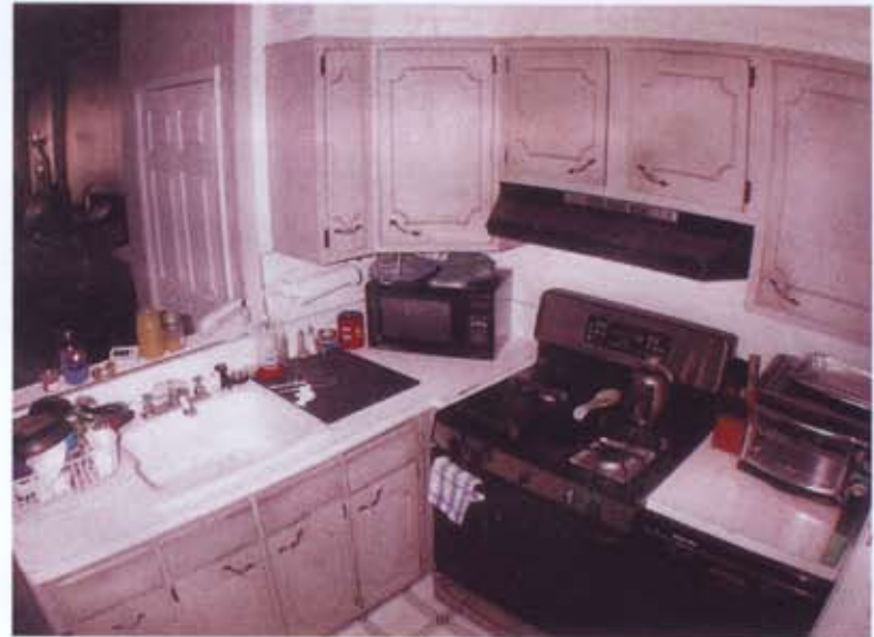
The Pierandozzi kitchen was in rough shape prior to the makeover. The floor was so pitched you could roll an egg all the way across it.
